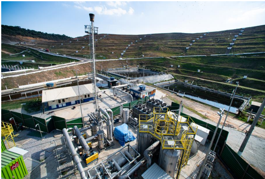
CTR Nova Iguacu 5000 Nm 3 /h open flare in 2018 and view of landfill site
