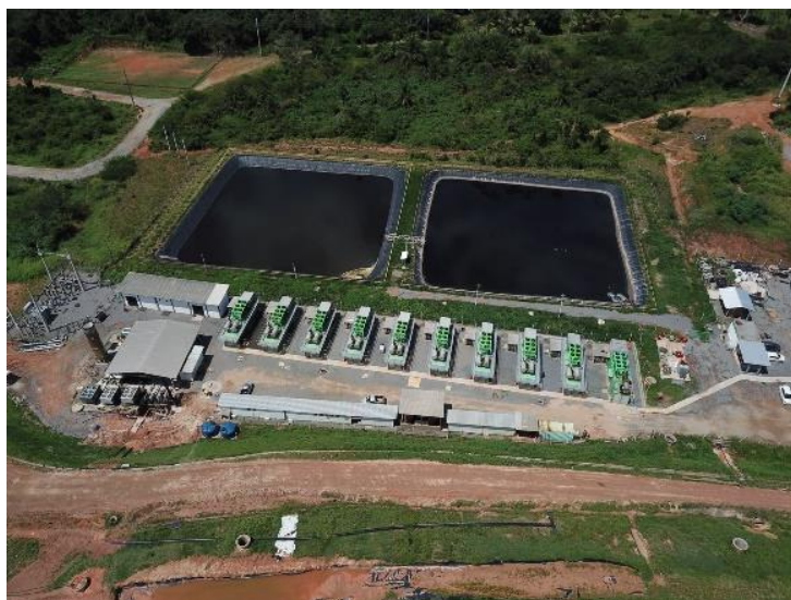
LFG Electricity Generation Plant in CTR Candeias landfill in 2021
