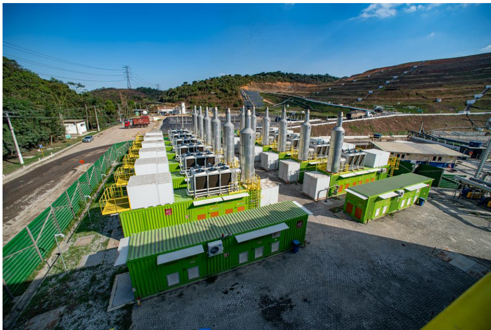
LFG Electricity Generation Plant in CTR Nova Iguacu landfill in 2021
